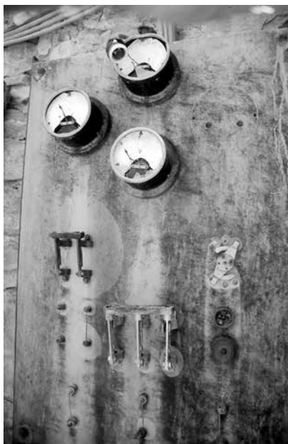
Panel de control — 2007
